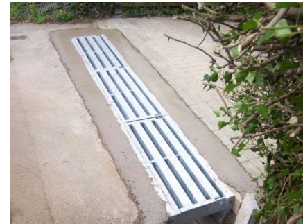
6. Installation Complete. NB. The outflow can run to either or both sides, or to a drain set in the base of the channel. In this case the outflow runs into a ditch.
