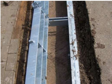
4. Stabilising the Units Bolt the units together and partially backfill with dry mix concrete to stabilise the units and to form the channel bed.
