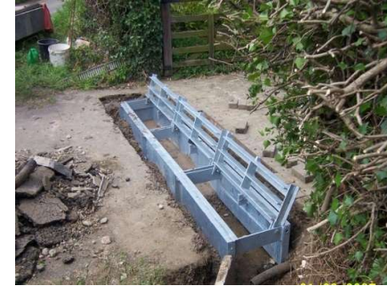
3. Bedding the Units In this case a dry mix has been used. The top of the units are set level with the road surface.
