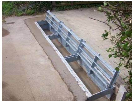
5. Finishing Off Back fill to form the channel and aprons using a normal C40 mix to BS 8500.
