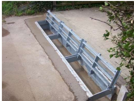
5. Finishing Off Back fill to form the channel and aprons using a normal C40 mix to BS 8500.
