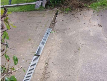
1. The Site Showing a typical installation; in this case replacing an inadequate slot drain.
