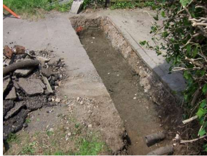
2. Excavate Pit and Prepare Sub-base Excavate to a depth of 750mm nominal. Eg. 300mm for the sub-base plus 150mm for the concrete bedding layer plus 300mm for the channel drain itself.
